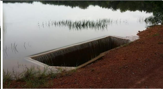
Estate A - Overflow as part of Water Management Plan to prevent flooding.
